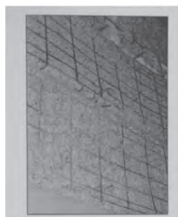
b) Surface spalling
