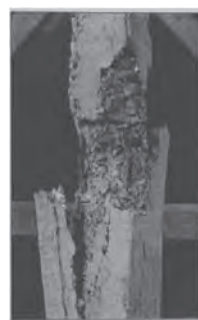
c) Corner spalling
