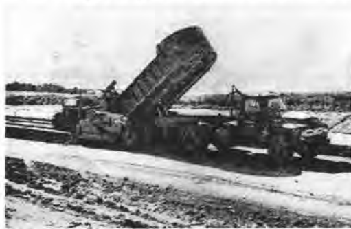
END-DUMP TRUCK feeds subbase material to self-powered Blaw-Knox spreader which lays material to a width of 14 ft and a depth of 11 in. After compaction depth is 8 in.
