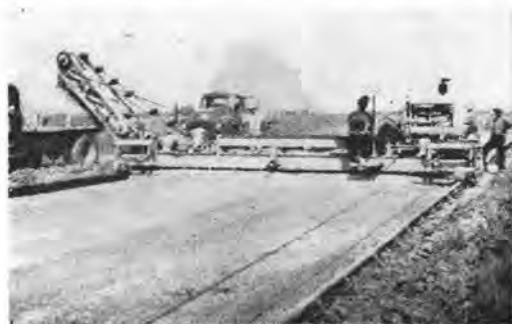
SUBGRADER removes excess material and conveyor loads it directly into trucks. This is faster, cheaper than usual method of depositing material in windrow for removal.
