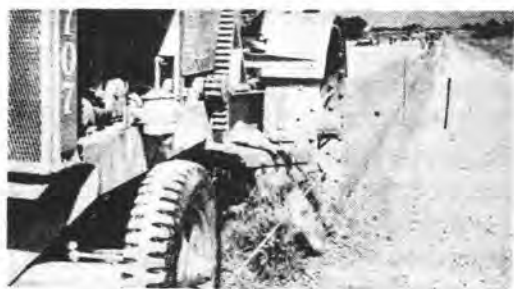
FORM GRADE is cut by Cleveland form grader at about 600 ft per hr. A bar connected to the blade rides on a stringline which indicates proper grade and alignment.
