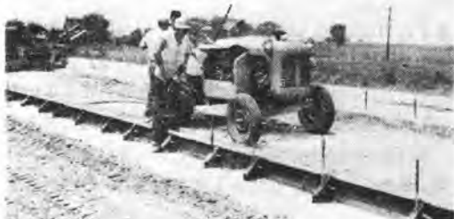
PNEUMATIC PIN DRIVER powered by a single-unit air compressor operating off a Le Roi tractor drives form pins. Blaw-Knox subgrade cutter follows a few feet behind (left).
