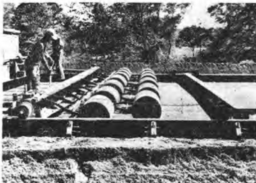
LAWN ROLLERS and scratch template attached to the rear of a mechanical subgrader make the final compaction and check subgrade elevation on section of Indiana Turnpike.
