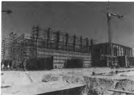
写真-2 SF-6 Switchgear Building
